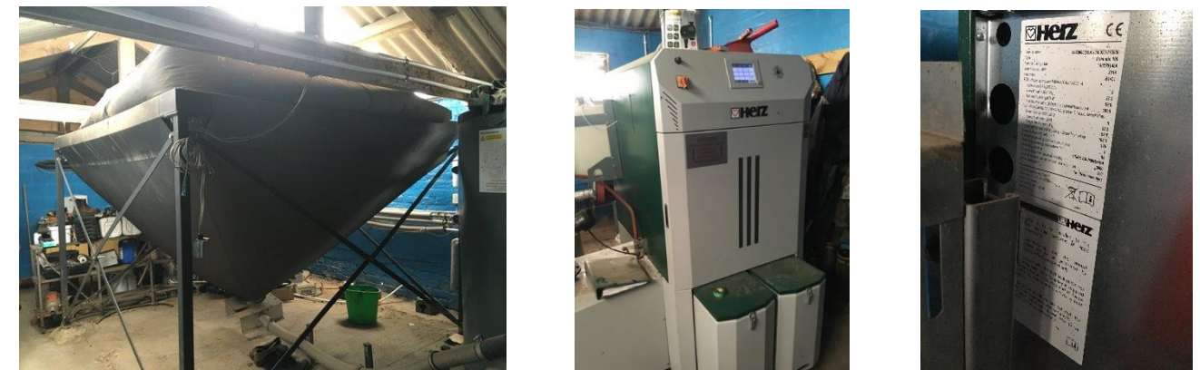
Figure 6—5 - 100kW Biomass Boiler & pellet hopper
